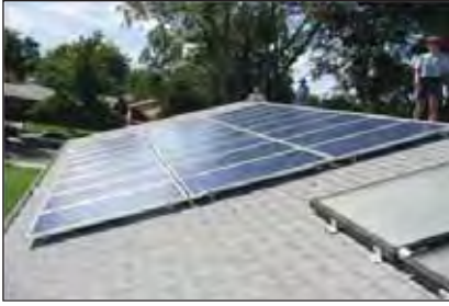
Roof-mounted, flush to roof solar electric array (Source: National Renewable Energy Lab [NREL])
